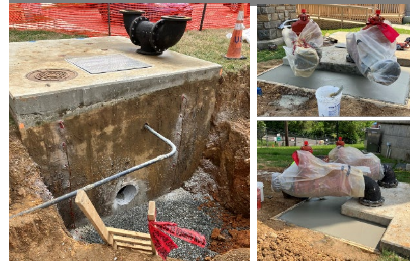
Emergency Booster Pumping – Ft. Reno PS
