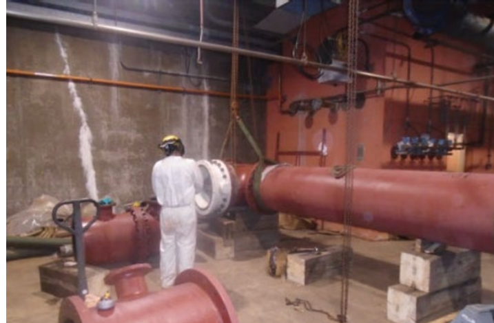
Reclaimed Final Effluent Pump Station Upgrades
