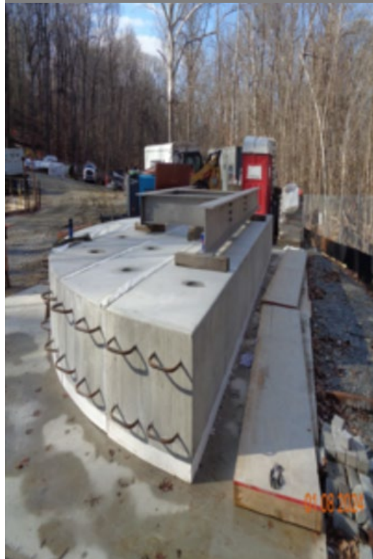
New MH31 Energy Dissipator
