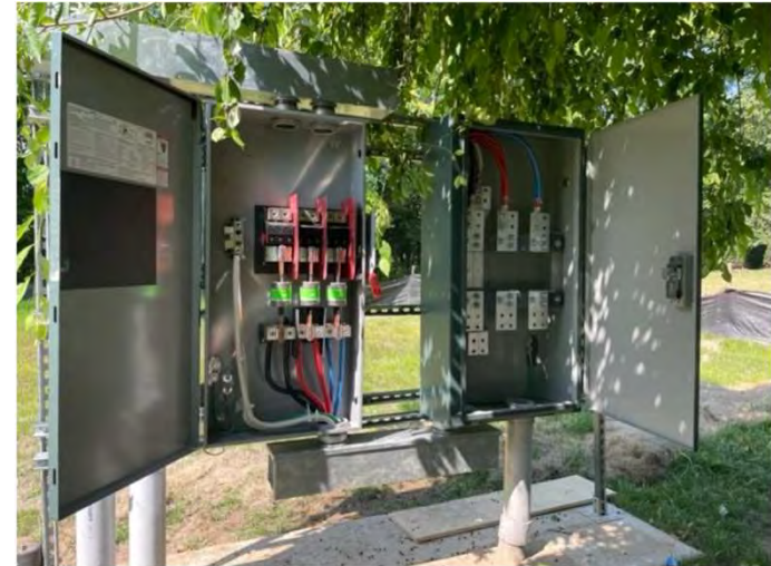
CSO-029 - Typical Electrical Gear Installation
