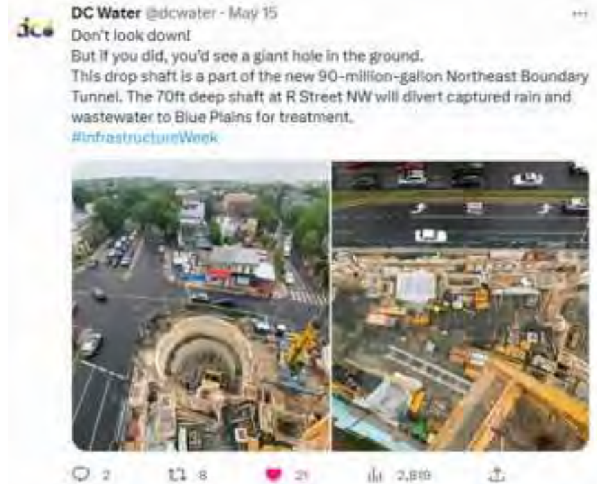
Twitter post of an aerial view of the R St NW construction site.
