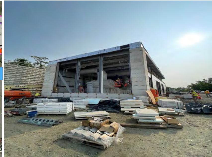
Ventilation Control Facility
