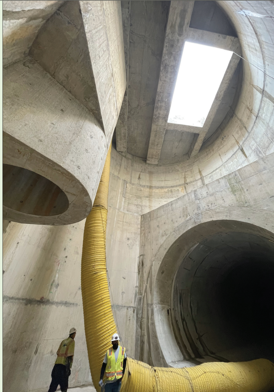
View from the bottom of the 38-foot diameter drop shaft at R Street NW. The large hole on the right is the entrance to the Northeast Boundary Tunnel.
