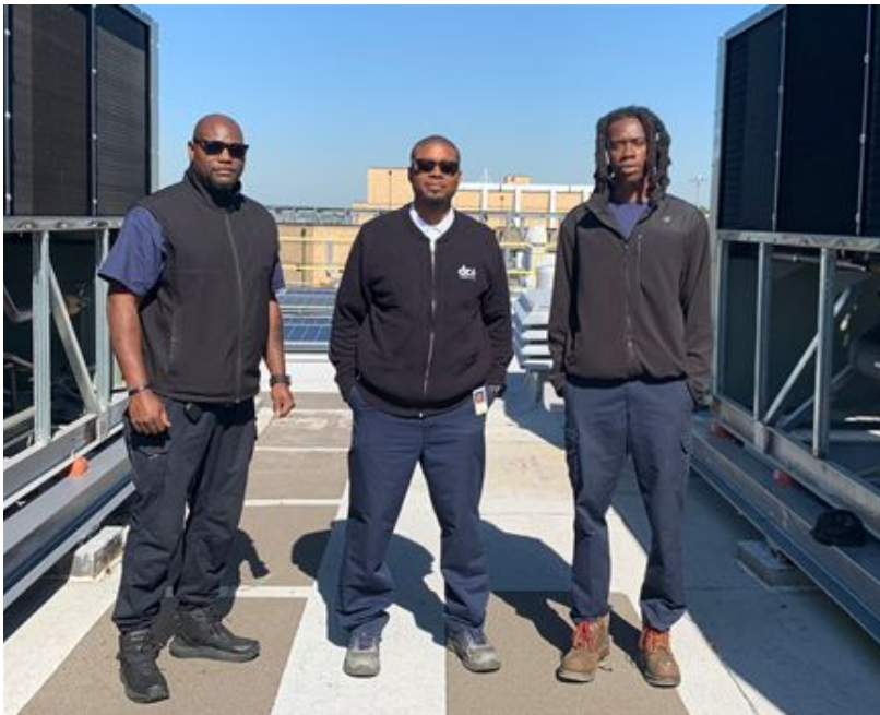
L-R: Harold Jusse , New AC Mechanic 10 (Started August 2023) William Shackelford , New HVAC Foreman (September 2023, Internal Recruit) Matthias Frazier , AC Mechanic 10 (DC Water Apprentice Program, Round 1 Graduate, July 2023) – Flanked by two new chillers for CMF Building, Blue Plains.
