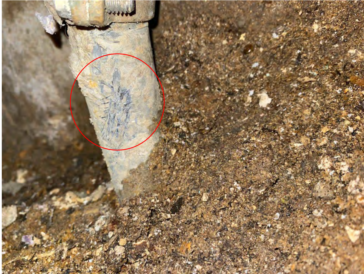
✓ Good 1 st Fitting Pic of Scratched Lead Pipe
