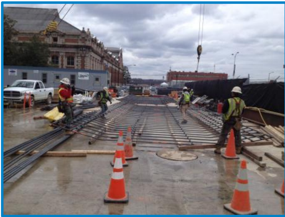
Photo 5-6: Main Pumping Station Drop Shaft Slurry Wall Rebar Assembly (Photo Taken March 1, 2013)
