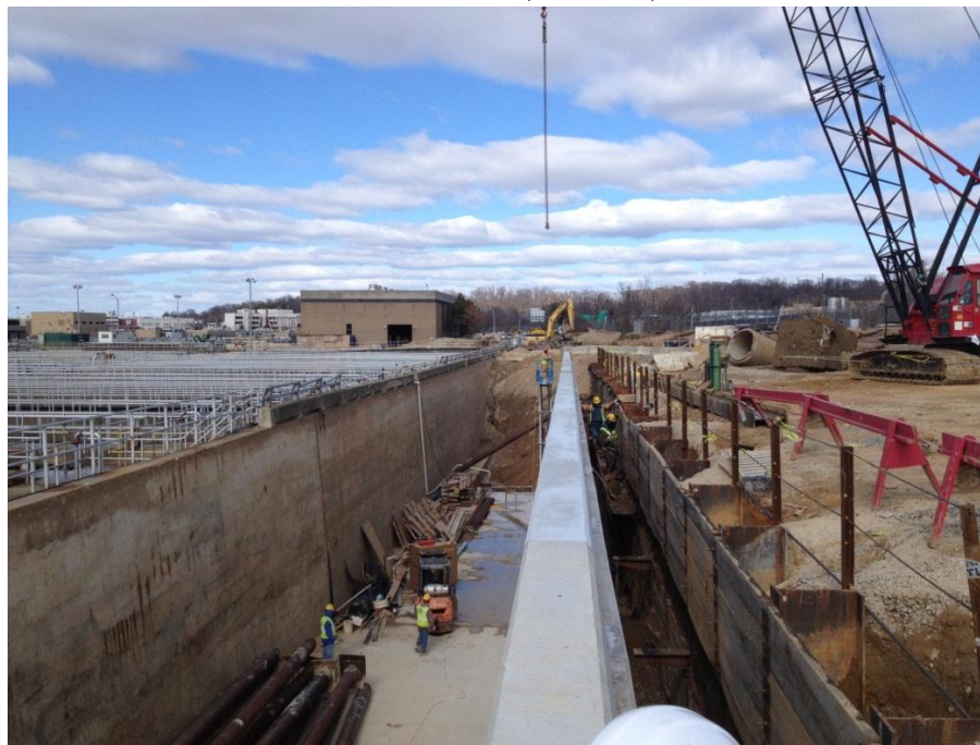
Photo 1 - Channel that conveys, mixes and adds supplemental carbon to nitrified mixed liquor. Under construction, March 8, 2013.
