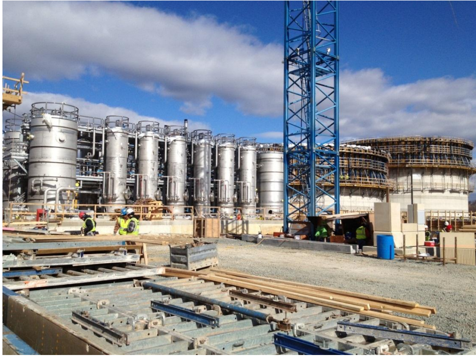
Photo 3 – Cambi Hydrolysis Process Trains (left) and Concrete Sludge Digesters (left) under construction. Photo taken March 8, 2013.
